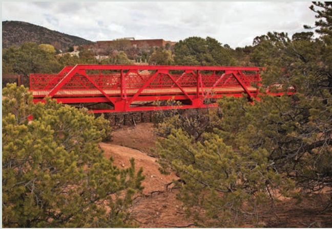
The hard-to-miss Kearny's Gap Bridge over the Arroyo de los Pinos connects the various gardens to one another.
