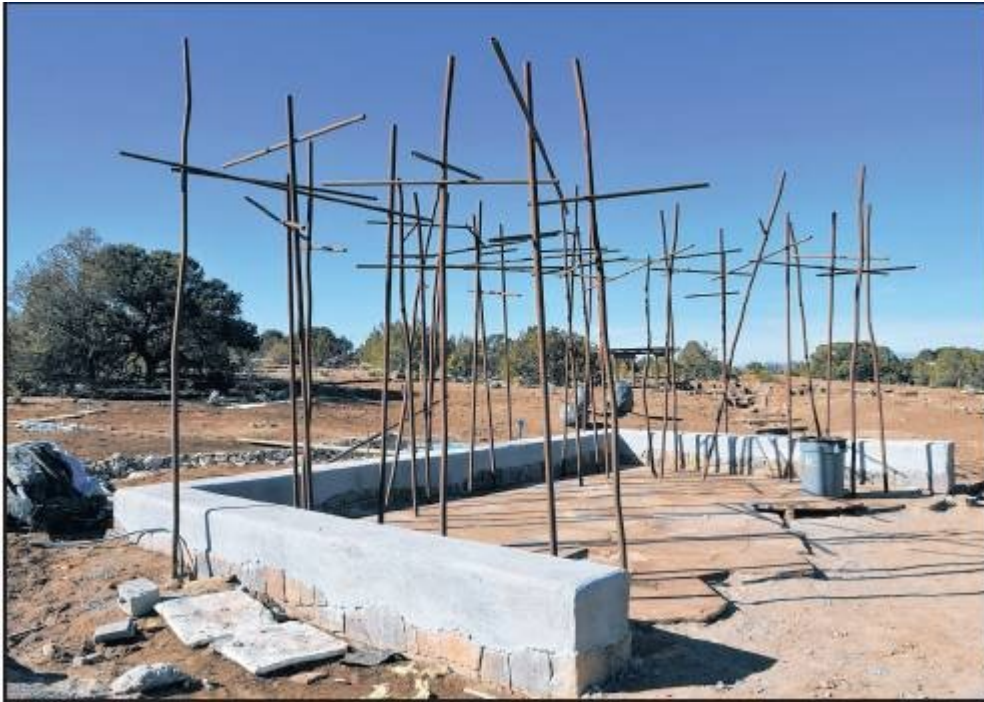
This arbor will support trumpet vines in the new Santa Fe Botanical Garden under construction on Museum Hill.
